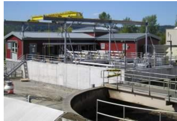
City of Duvall, WA: MBR replaced and expanded existing conventional system, using existing tanks for part of the biological process
