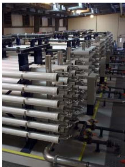
Municipal RO Installation
