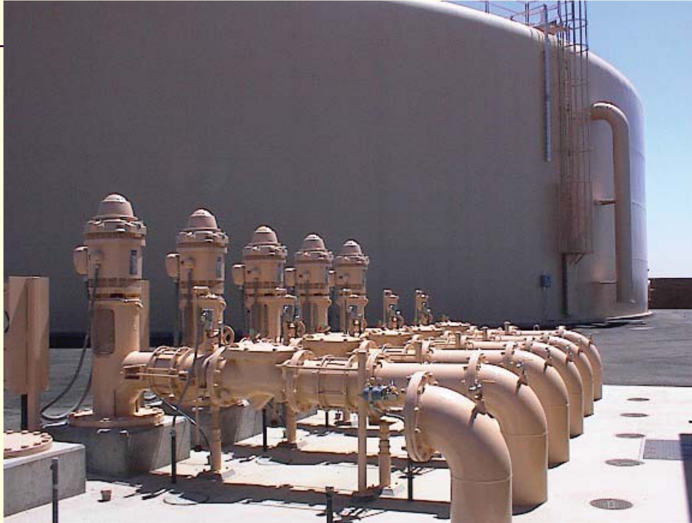
water pumping station
