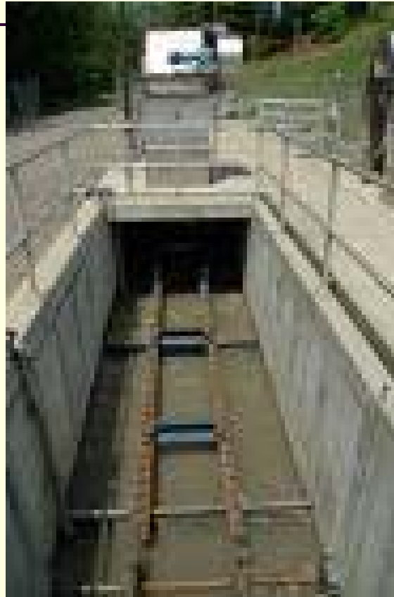
Grit Removal Channel
