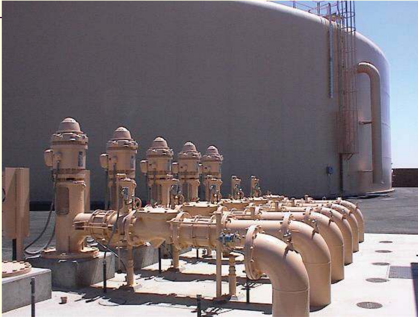
Distribution pumping station
