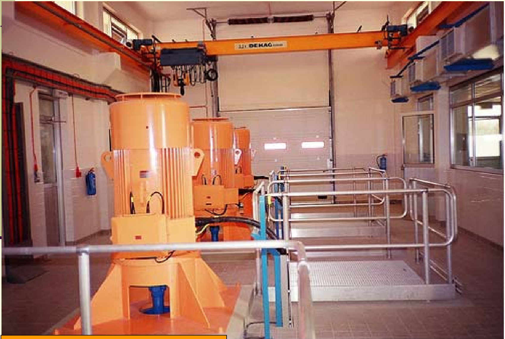
Fig. 5.10 Dry room for dry pumps
