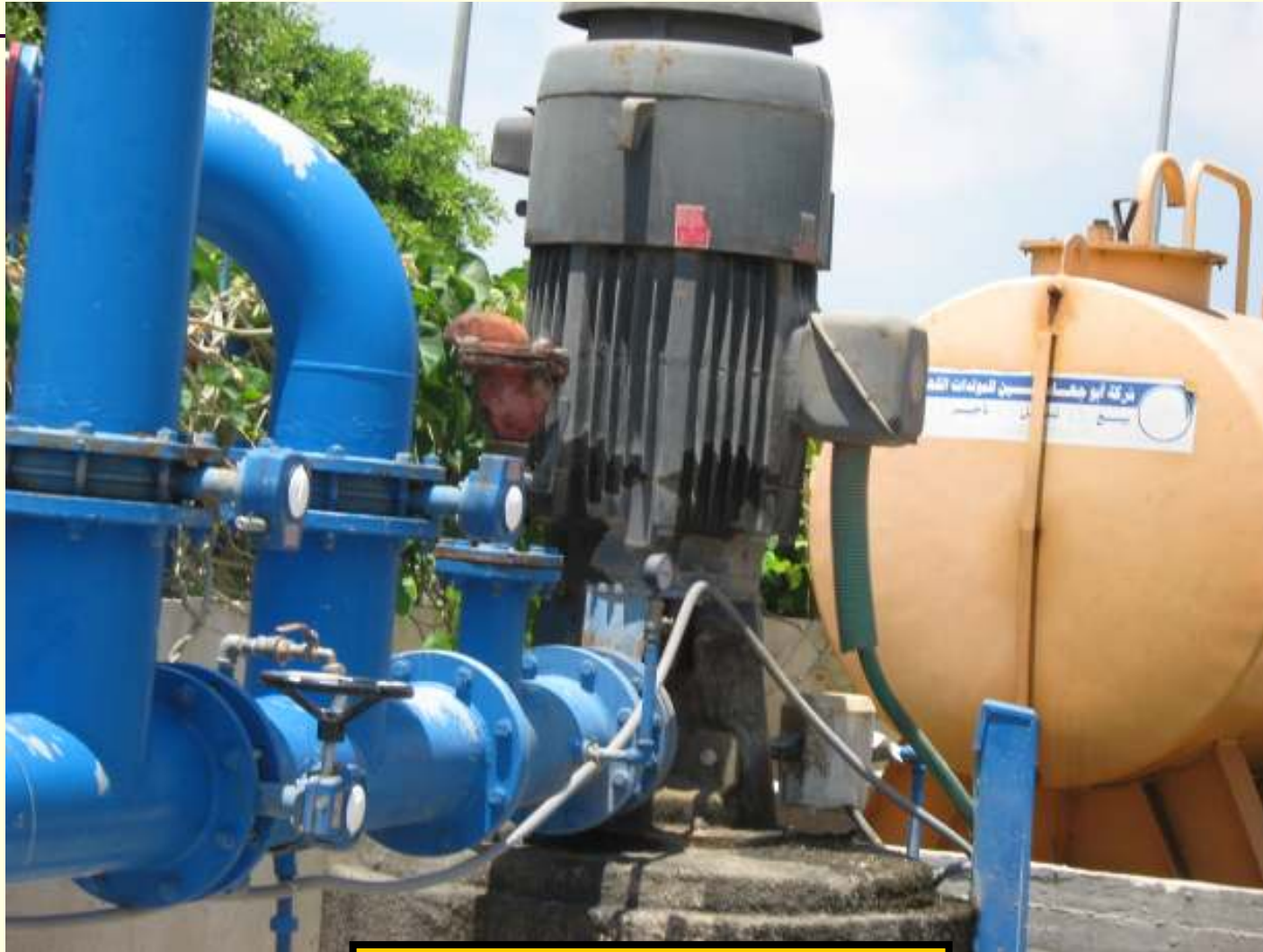
Vertical dry motor installation
