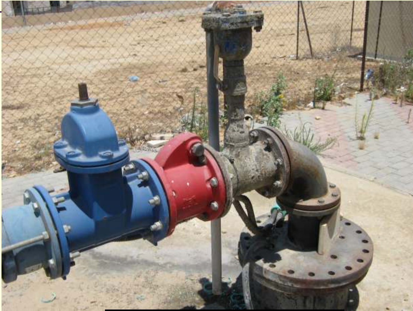
Submersible type motor installation
