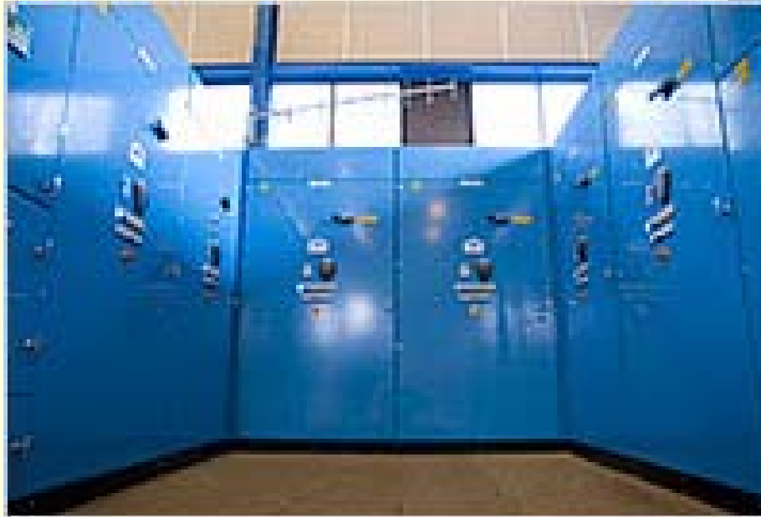
Pumping station Control Panel
