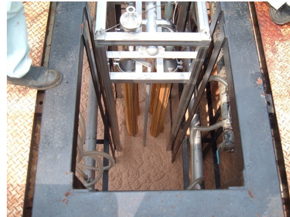
Soaking Asahi-kasei MBR rack in aeration tank
