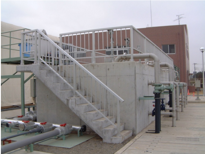
(a) Cooperative influent tank
