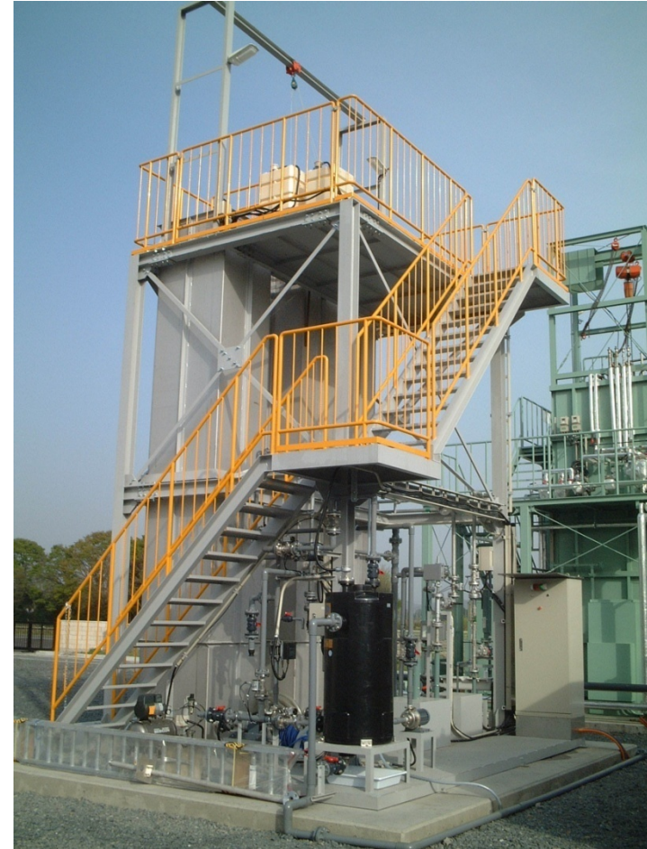
(b) Asahi-kasei MBR Pilot Plant
