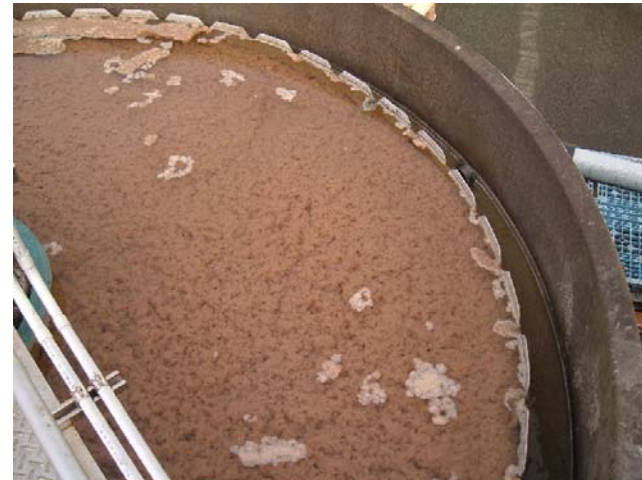
Carry over of activated sludge
