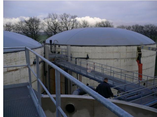
Methane fermentation tank
