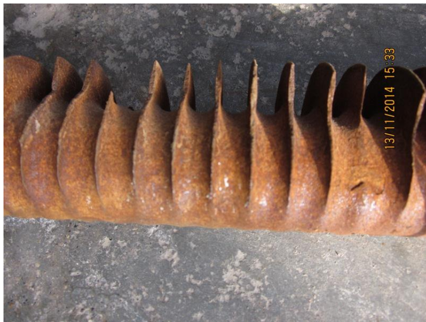
Figure 1: severe acid corrosion of economizer tube
