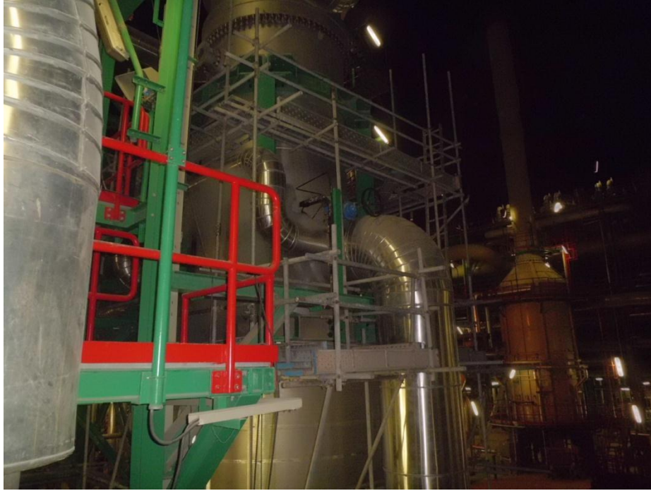
Figure 1: Leaking Process gas bypass valve of E0309
