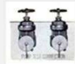
Pump Test Connections
