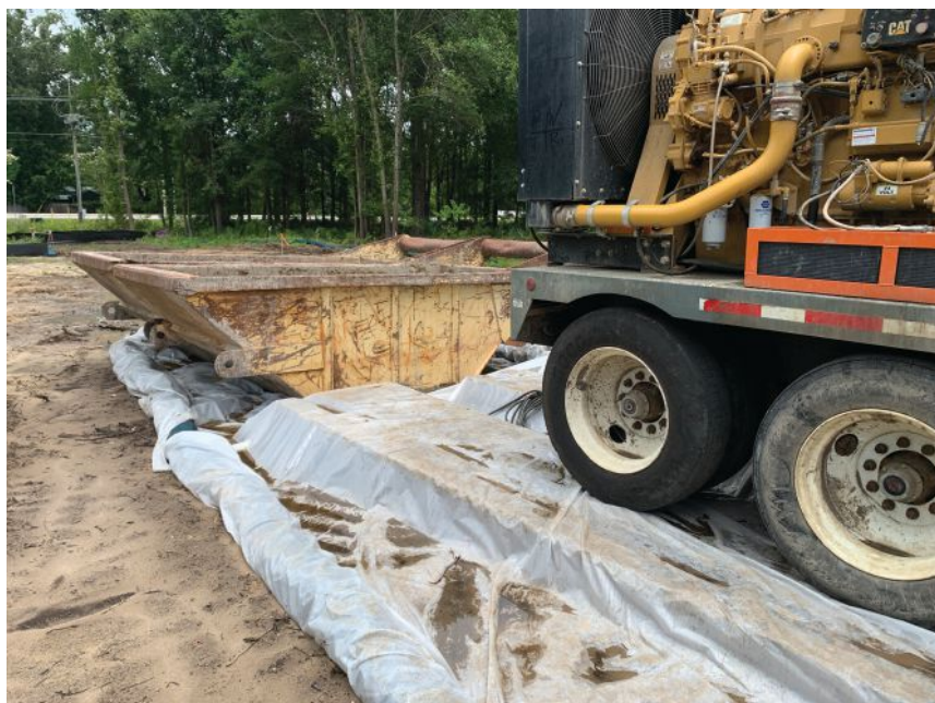
Erosion controls and secondary containment prevent impacts and can easily be inspected and maintained.
