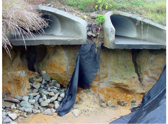
Even with the mostly flat slopes typical of the area, scour at pipe outfalls is still prevalent.
