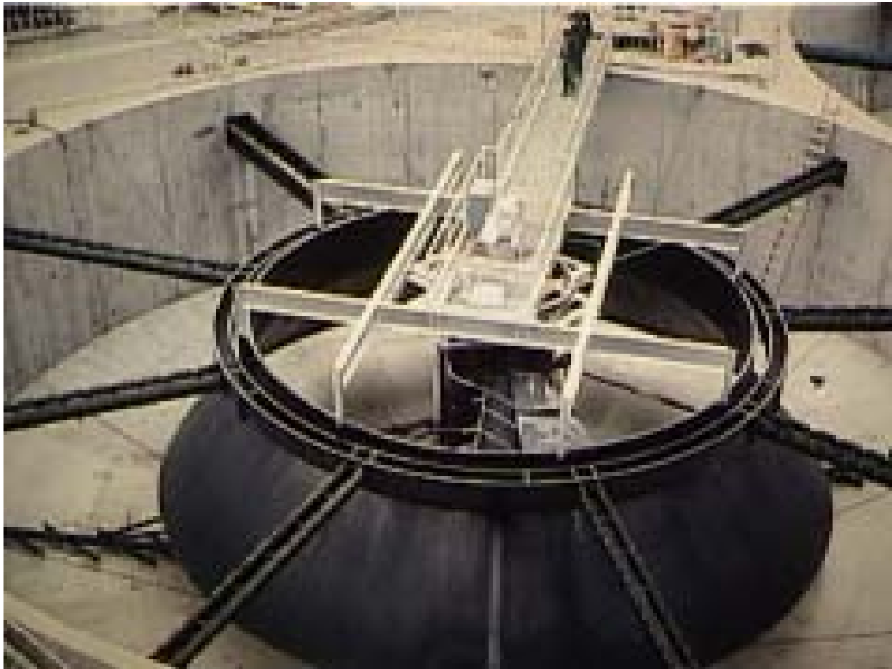
Figure 3.18 : Solids Contact Flocculator Clarifier
