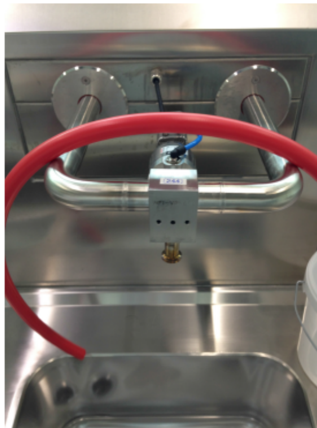
Sink with sterilized hose (e.g. with rinsing)
