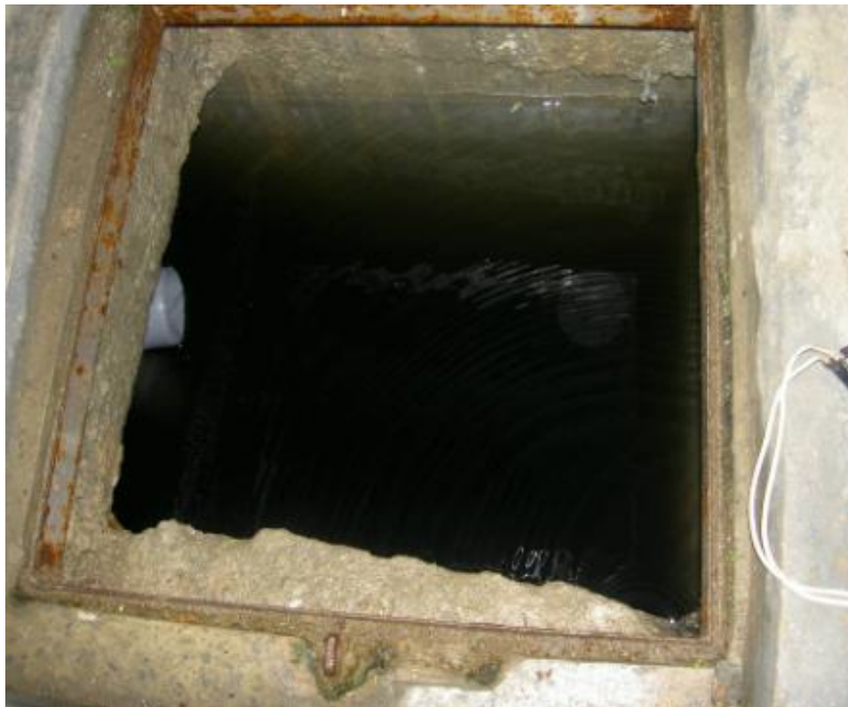
Water tank: 9000 liters
