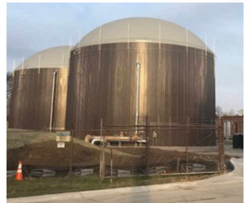
Anaerobic digesters at the Kenneth W. Hotz Water Reclamation Facility
