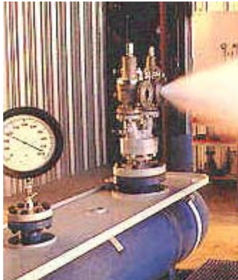
Figure 6.5: Pressure Testing a PSV/PRV
