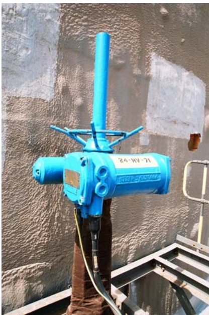
(a) Motor-actuated Gate Valve
