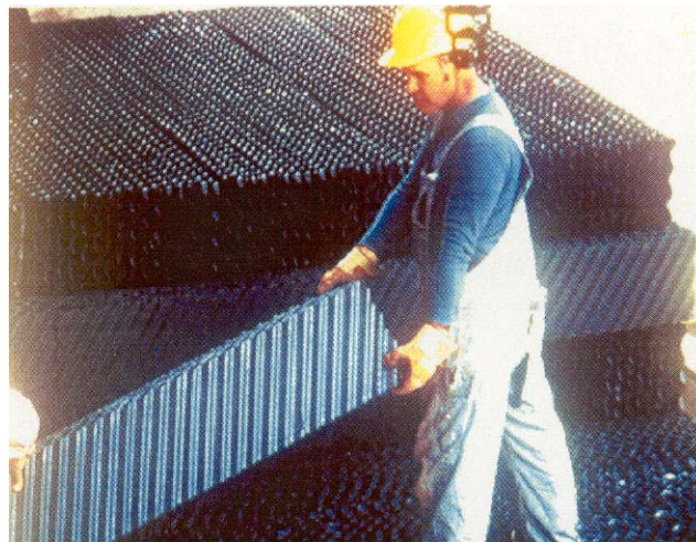
Figure 4-11. High-Efficiency Cooling Tower Film Fill
