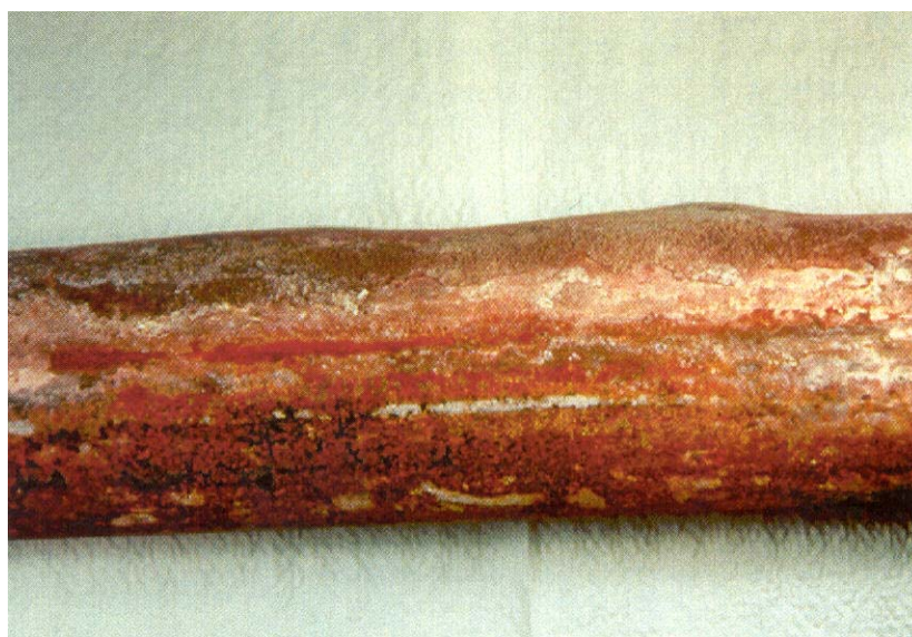
Figure 3-7. Metal Fatigue on Boiler Tube
