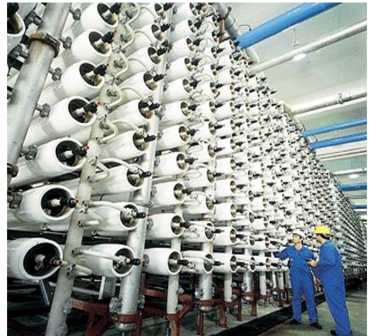
LARNACA SWRO WATER DESALINATION PLANT, CYPRUS (54,000 m 3 /day)
