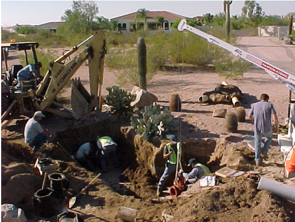
A cross completely blown out. A major job. Good thing it wasn't under the blacktop.
