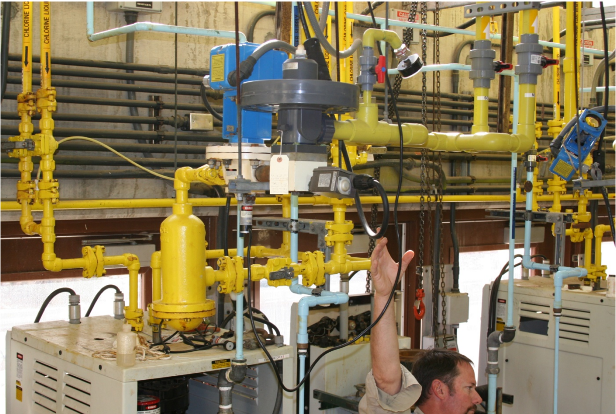
Chlorine gas piping.
