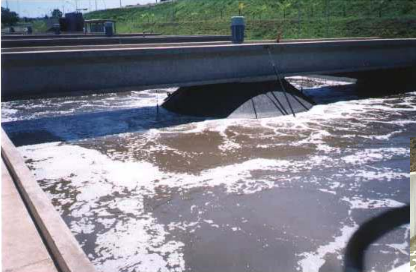
Surface Aerators in Aeration Tank
