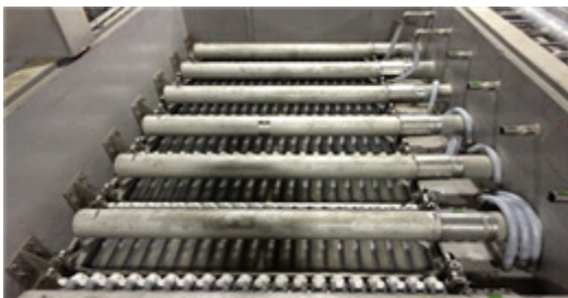
UF Pre-treatment separation membrane
