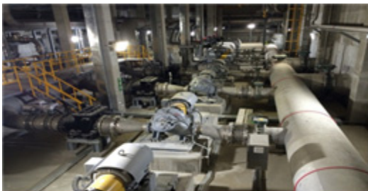
Reused water supplying facilities
