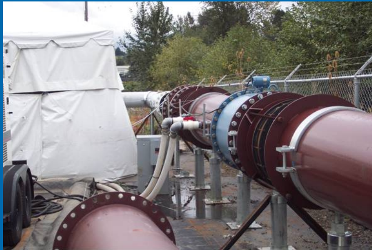
Inlet piping showing mixers, magnetic flow meter, MS2 and LS injection, 90 degree bend
