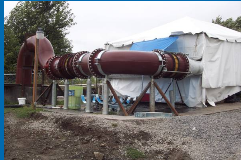
Outlet piping with discharge
