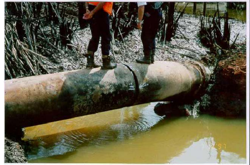
Pipe rupture location
