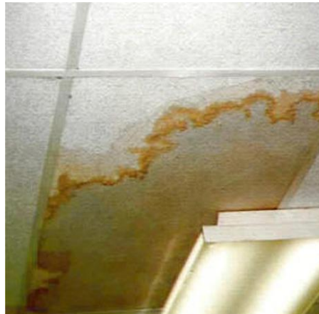
Water damage on ceiling
