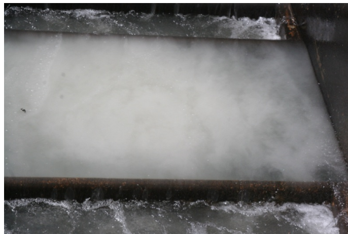
Backwashing a filter.
