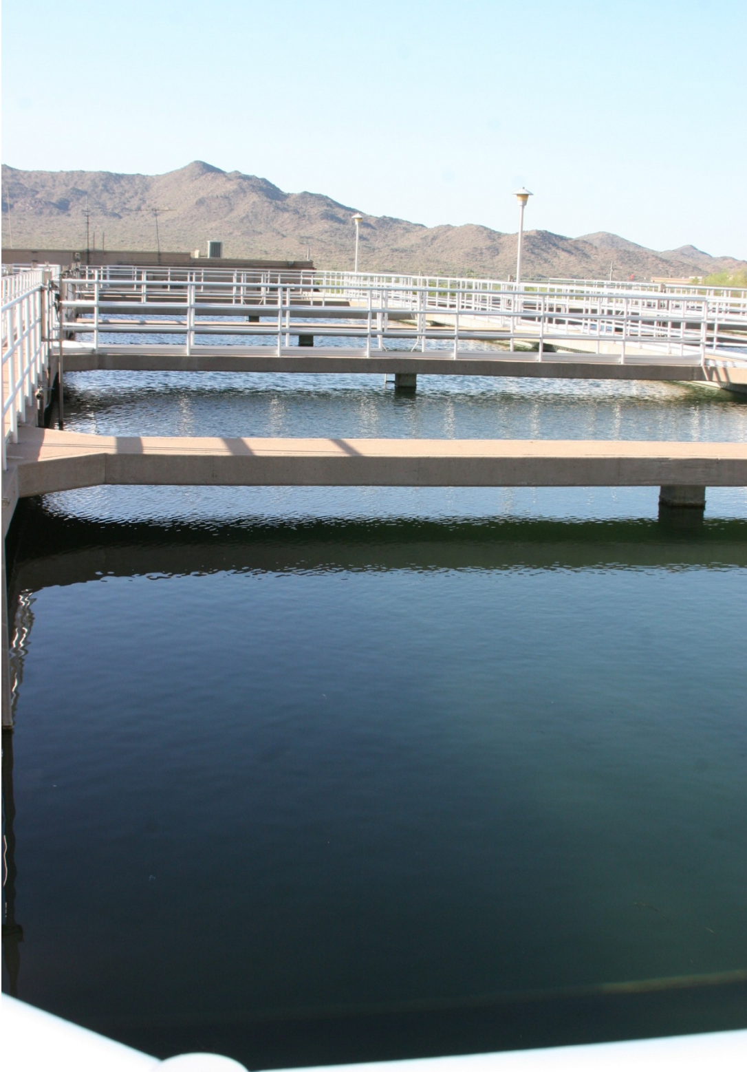
This photograph overlooks the flocculation basins at a water treatment plant.
