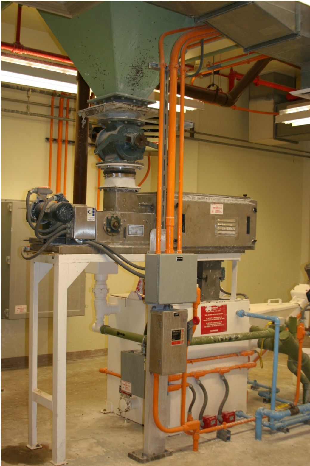
Some plants use Lime as a coagulant or for softening. This is a lime slacker.
