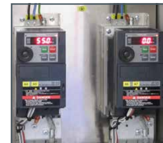
Frequency converters for controlling the pumps
