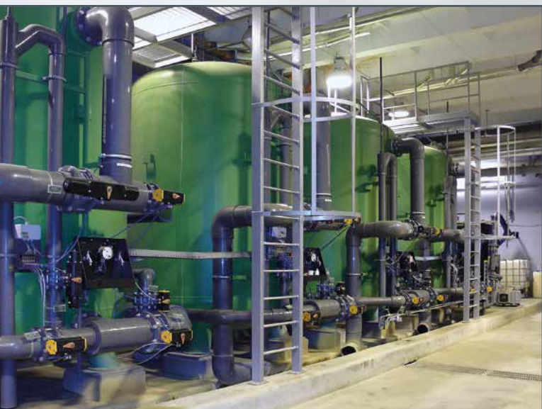
Continuous-flow adsorber in a water treatment plant
