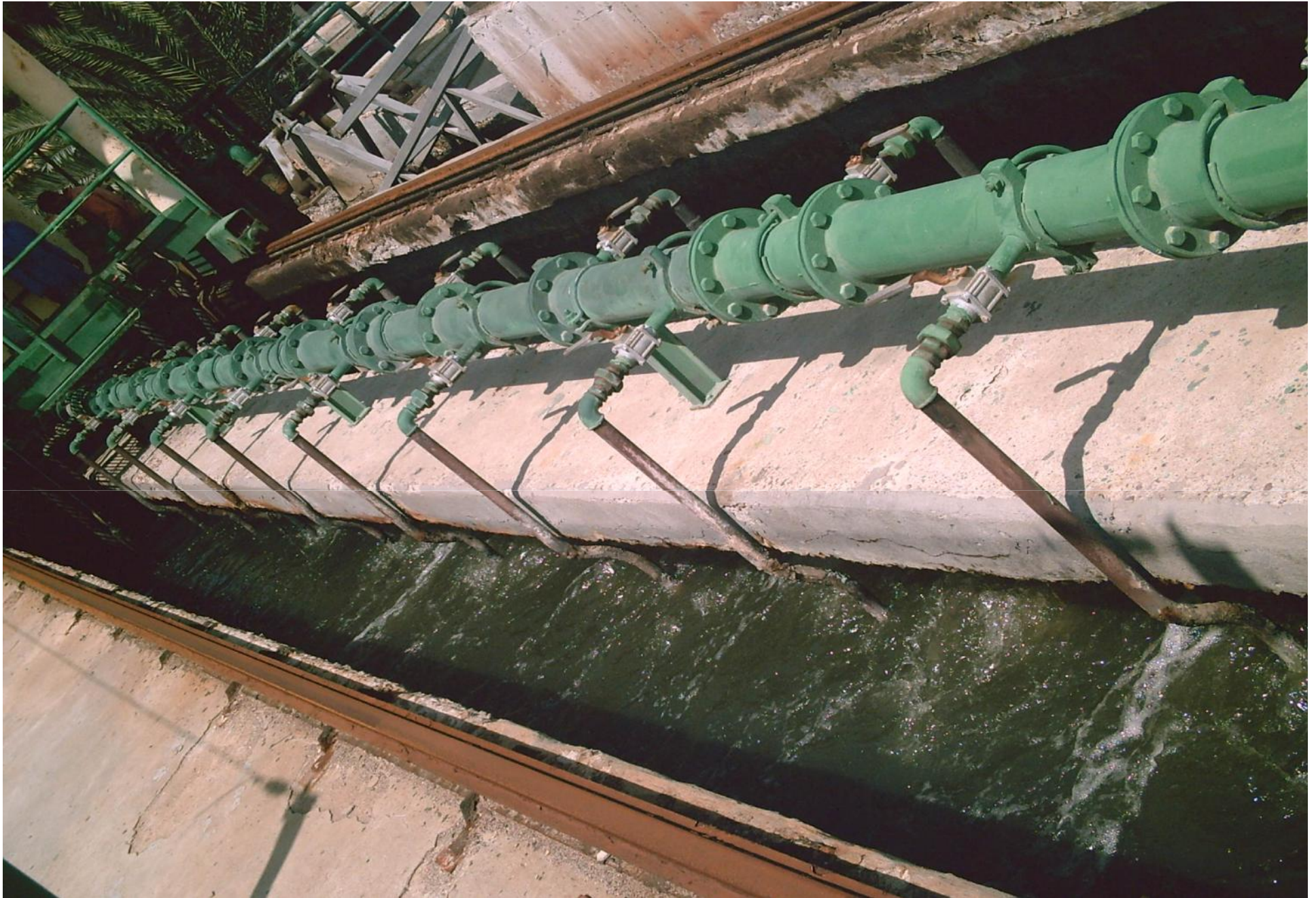
Compressed Air Pipe
