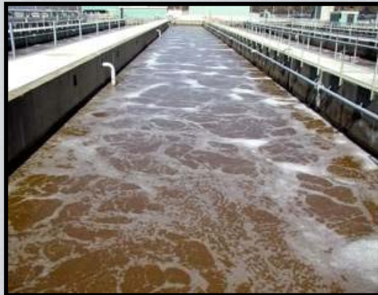
Diffused Aeration System
