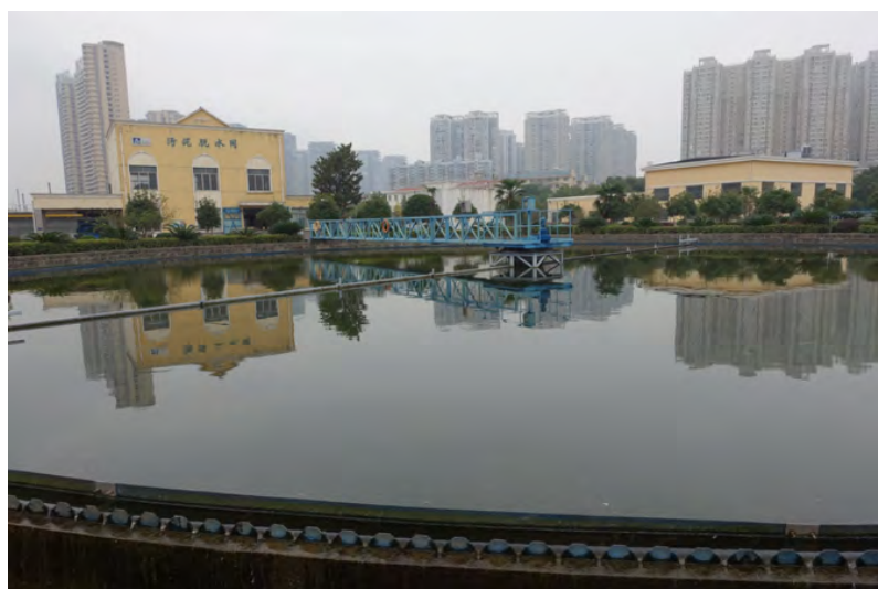
Figure 47: A photo of a circular clarifier
