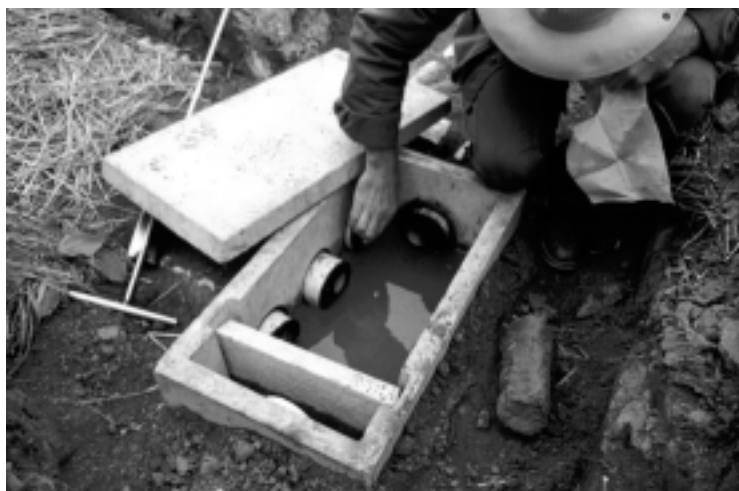
Figure 4-8. Distribution box with adjustable weir outlets
