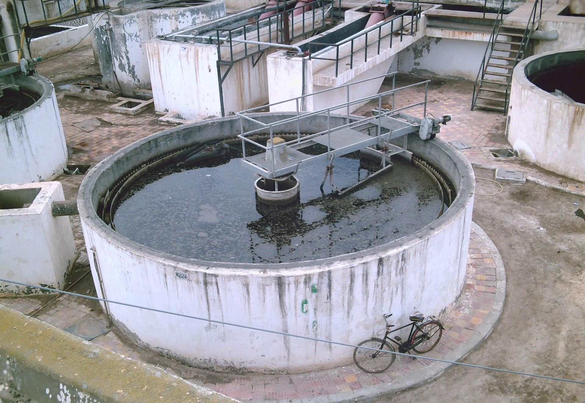
Final Sedimentation Tank
