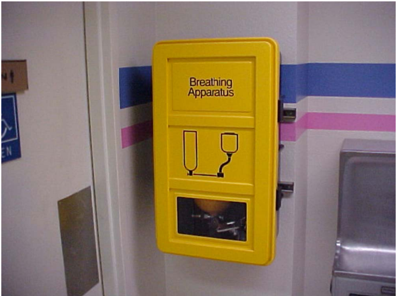
SCBA Storage Box
