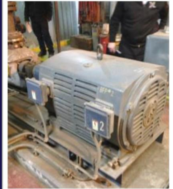
Boiler Feed Pump 2
