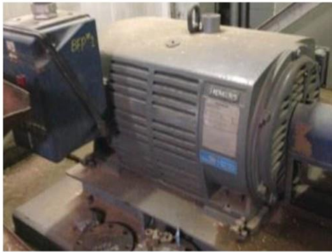
Boiler Feed Pump 1
