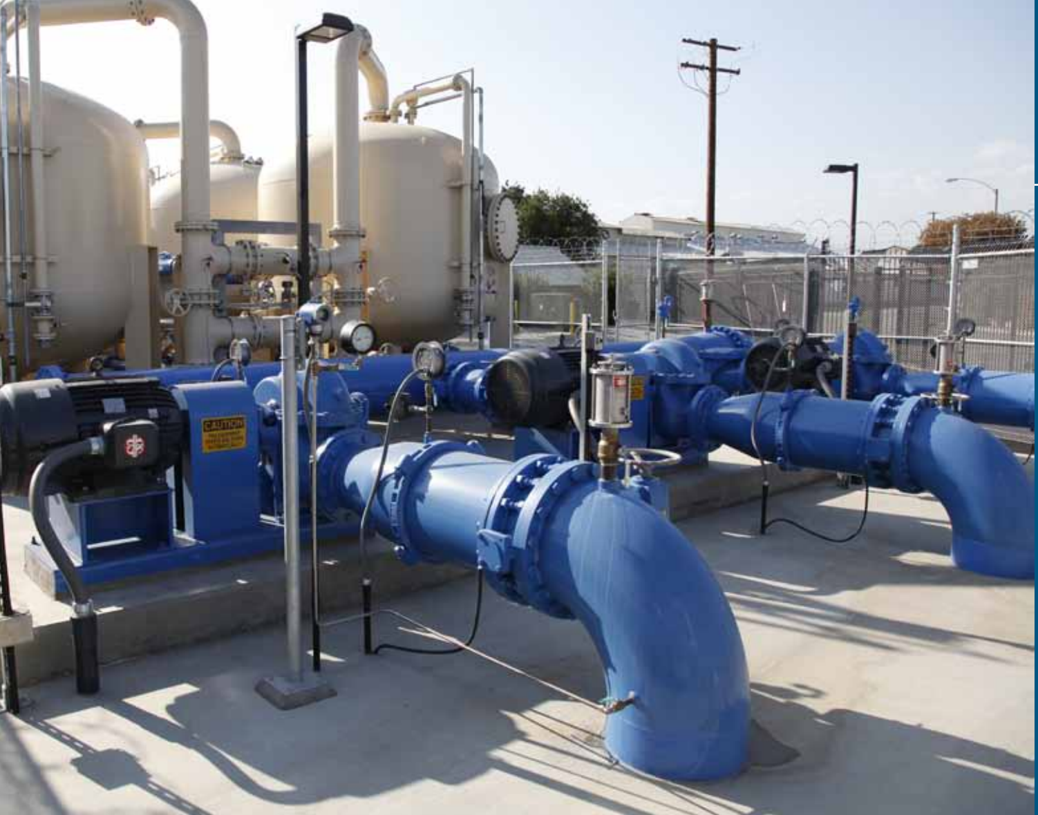
The Montevina WTP pumping system delivers high quality water from the foothills south of Los Gatos, California.
