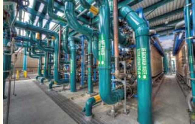
RO membranes process equipment.
