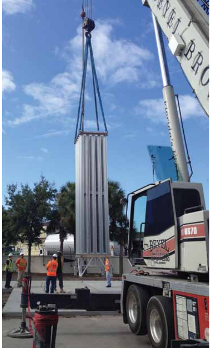
Installation of a liquid oxygen system — one component in treating water to high quality standards.
