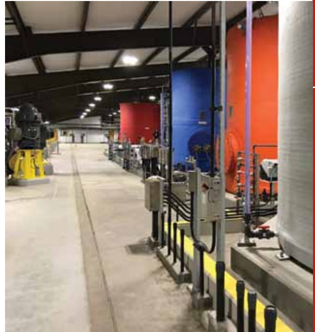
A 52' deep underground storm and wet weather station in southwest Florida with 27 mgd pumping capabilities.
