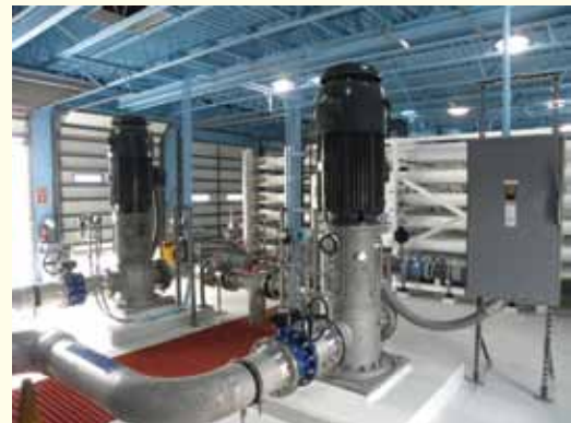
Newly renovated and upgraded reverse osmosis system skids
