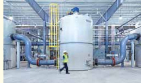
Pretreatment system for sediment at Onondaga Lake.
