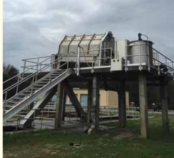
The new headworks system receiving wastewater influent for preliminary treatment
