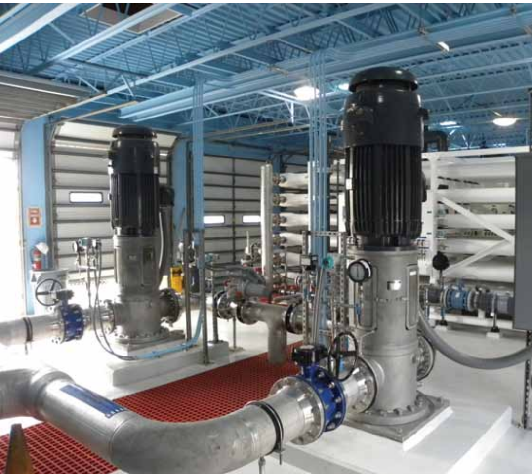
The newly renovated and upgraded reverse osmosis system at the Venice, FL, 4.5 mgd water treatment plant enables the system to meet the existing TDS and flow conditions.
