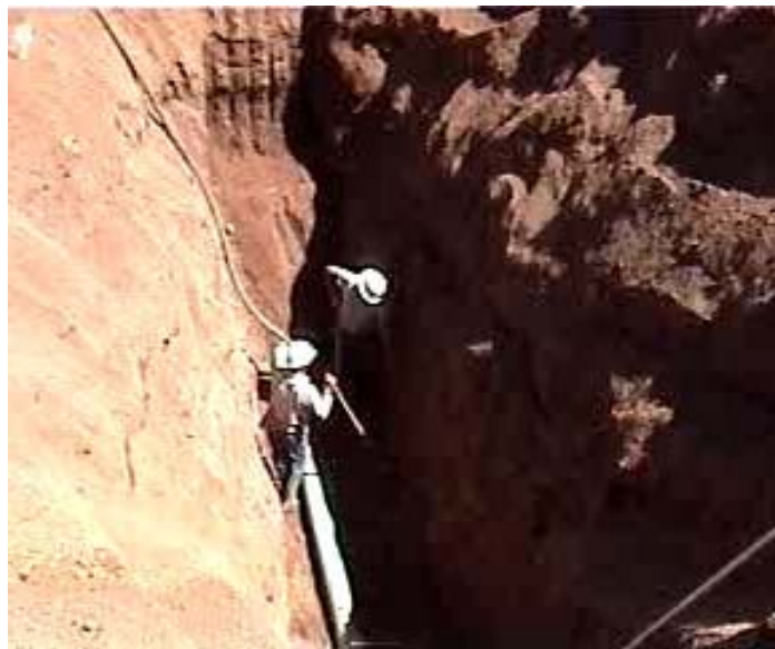
Death trap, no way out. No shoring.
