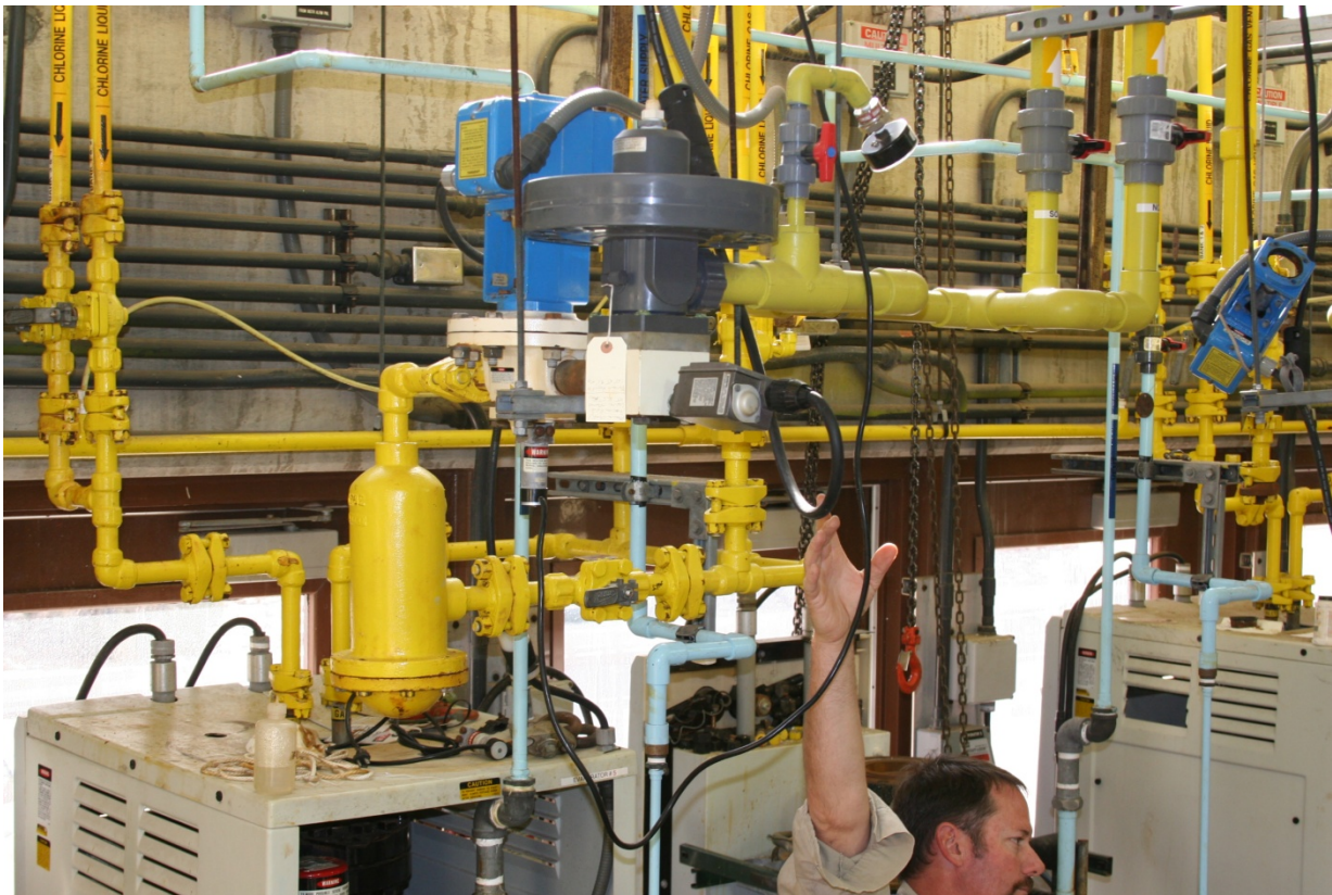
Chlorine gas piping.
