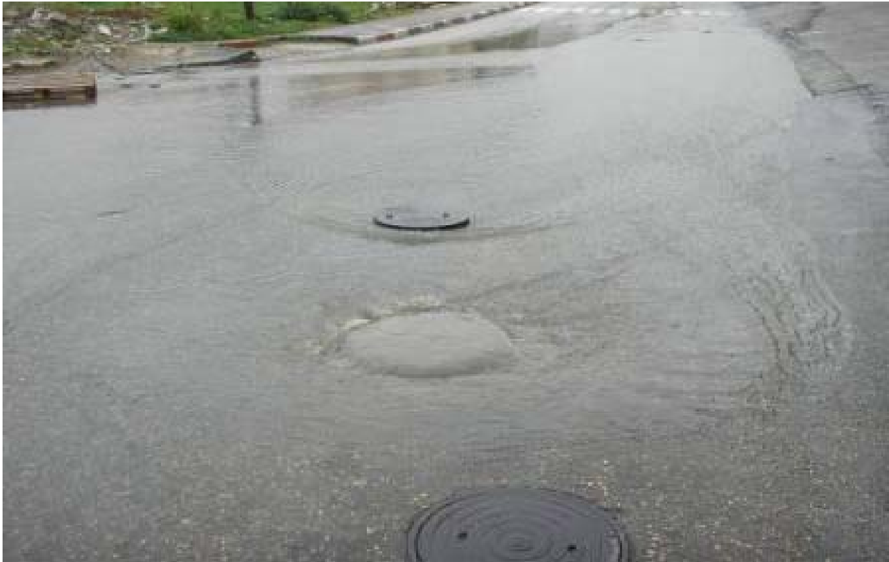
Mixed “Wastewater and Stormwater” flows out of a sewer manhole (Infiltration into Sewers)
