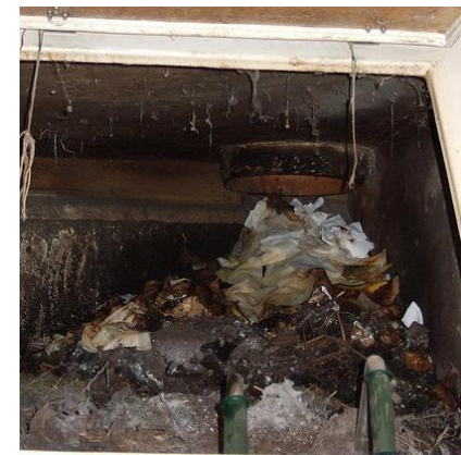
Right: composting chamber for excreta, toilet paper and organic household waste in Hamburg-Allermöhe, Germany. Source: SUSANA on Flickr (2012)
