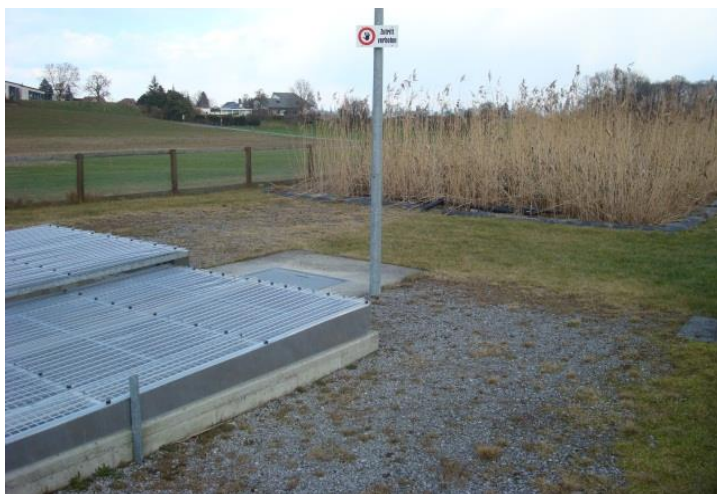
On-site treatment system in Switzerland for 36 p.e. Covered compost filter (left), covered pump shaft and vertical flow constructed wetland as a last treatment step (right). Source: STAUFFER (2009)
