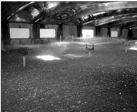
Intermittent sand filter (Secondary Treatment)
