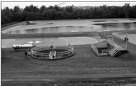
Aerated lagoons are secondary treatment processes.
