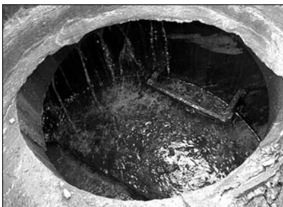
Groundwater infiltration makes efficient treatment difficult.
