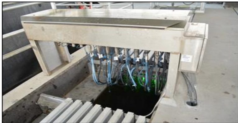
Figure 4-6 Disinfection (UV) at the Valrico Plant
