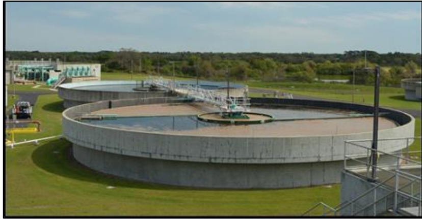
Figure 4-5 Secondary Treatment (Clarifiers) at the Valrico Plant
