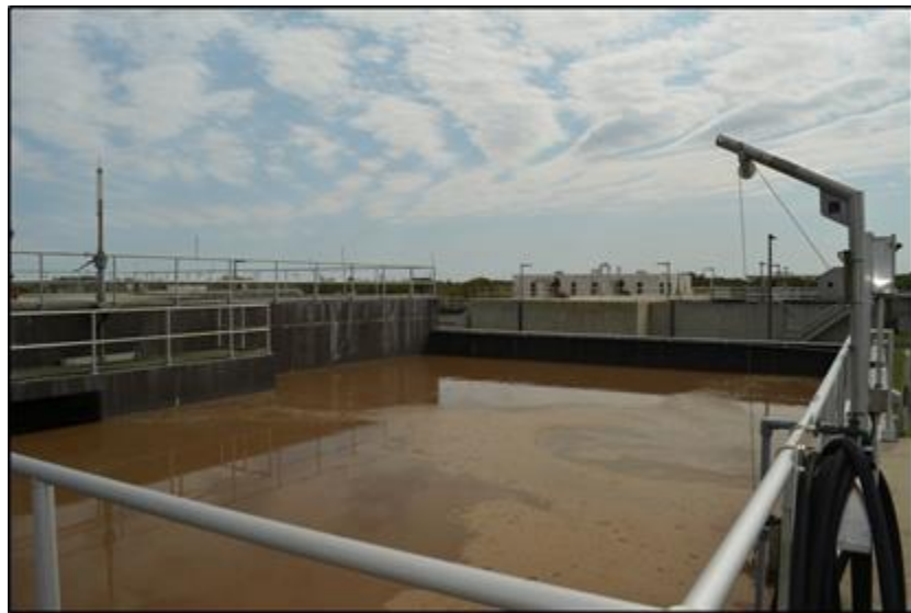
Figure 4-3 Secondary Treatment (Anoxic Basin) at the Valrico Plant
