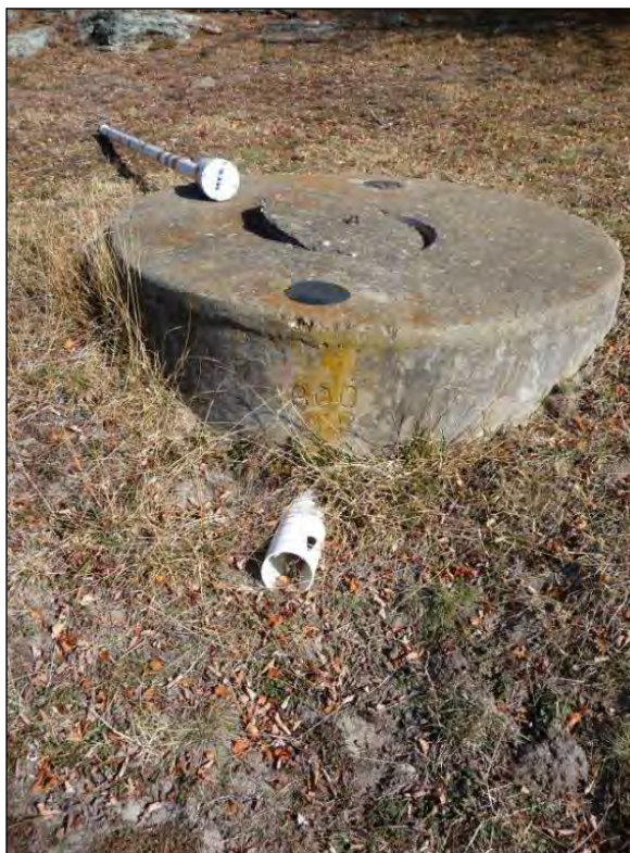
Figure 3.7 Outlet pipe discharging directly onto open ground
