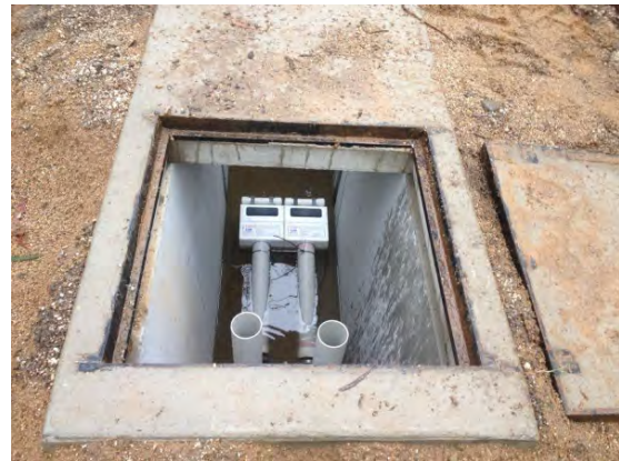
Figure 10.4 Flout in dosing chamber
