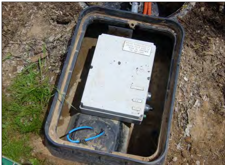
Figure 5.8 An electrical box that was flooded
