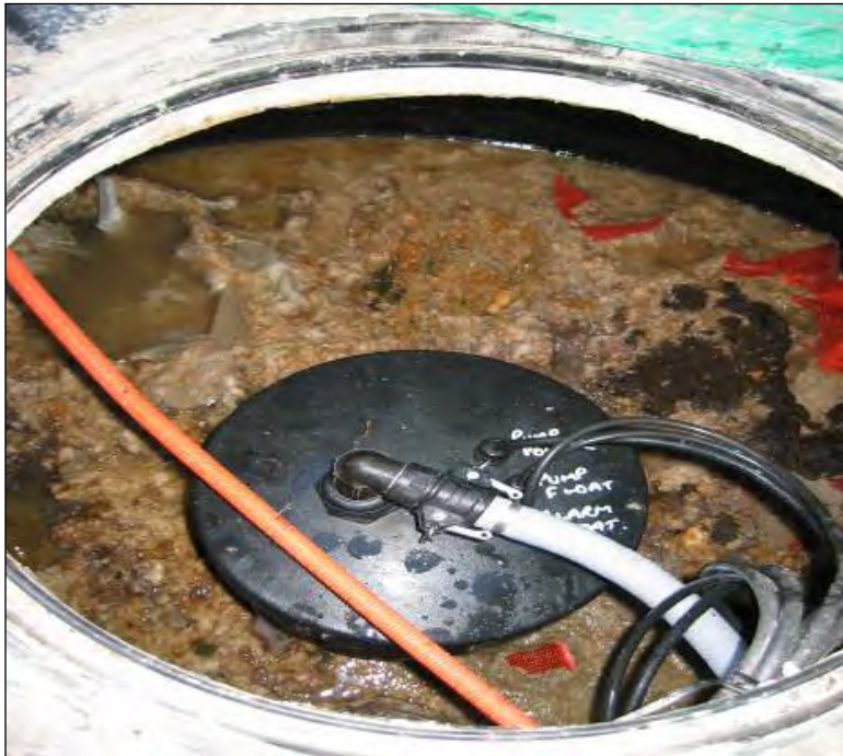
Figure 5.10 A flooded system due to pump failure
