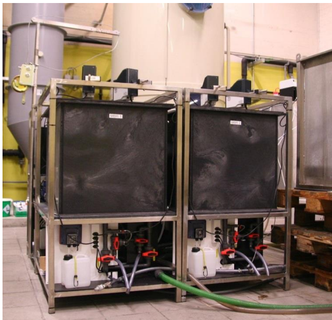
Figure 3.3 – Photo of the PAC + UF pilot plant
