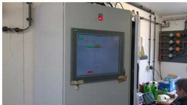
Figure 2.3: Photographs of the PAC-CMF pilot setup operated at WWTP Almelo.
