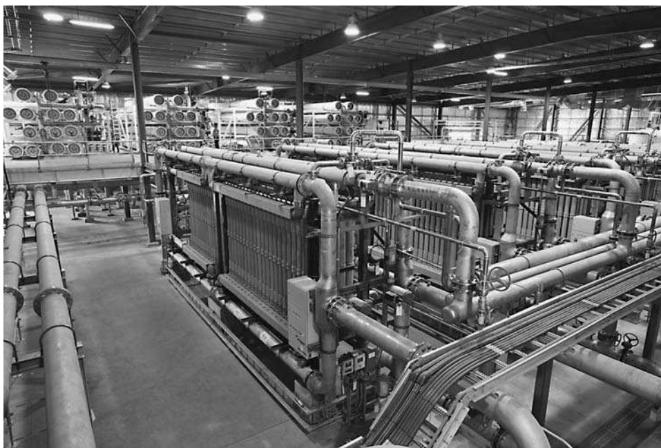
FIGURE 12.3 Pressurized MF system with vertical membrane elements.
