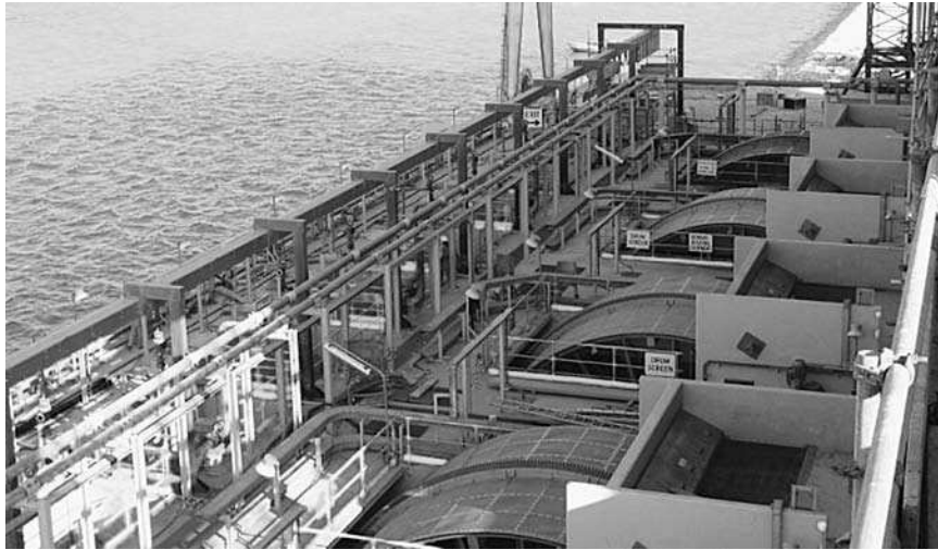
FIGURE 5.2 Fine intake screens.
