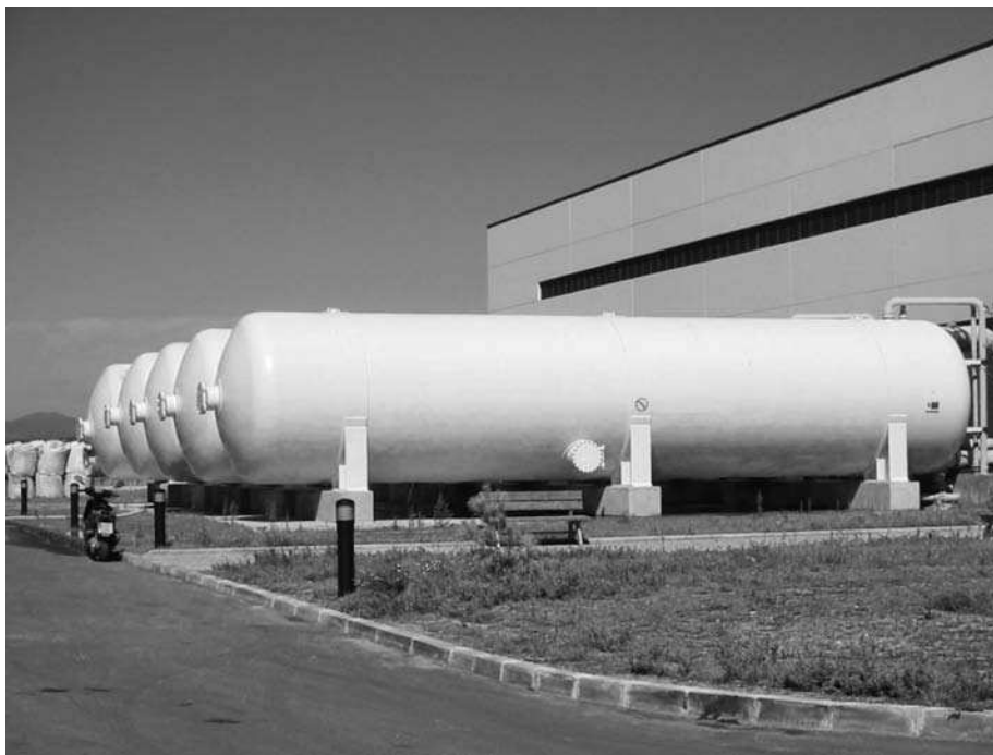
FIGURE 11.5 Horizontal pretreatment pressure filters.
