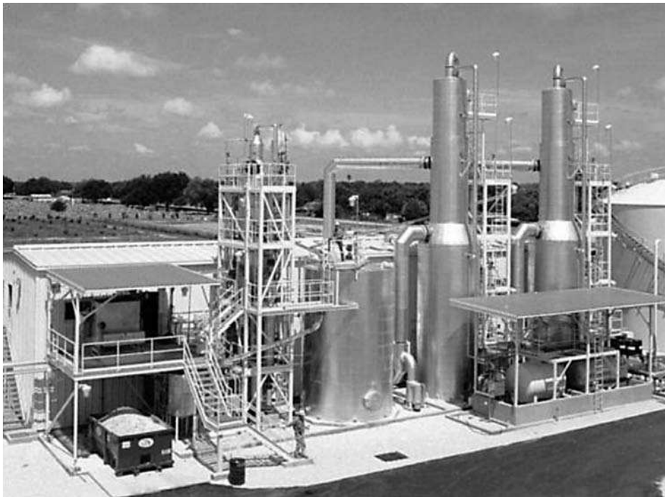
FIGURE 16.51 1000 m 3 /day (0.26 mgd) evaporator-crystallizer.
