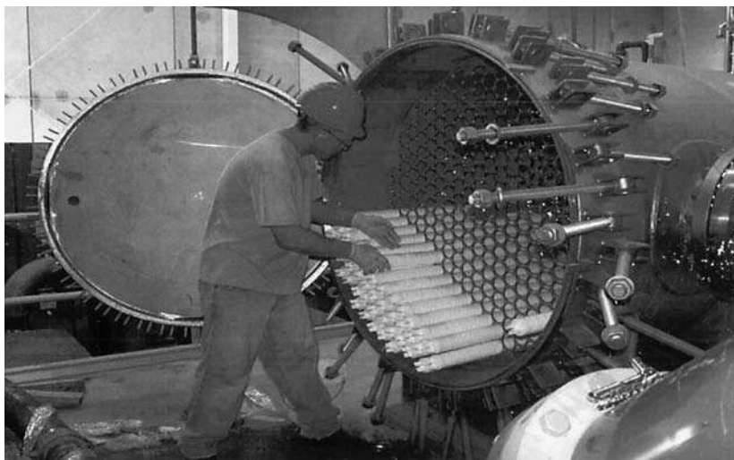
FIGURE 8.15 Cartridge filters installed in a horizontal vessel.
