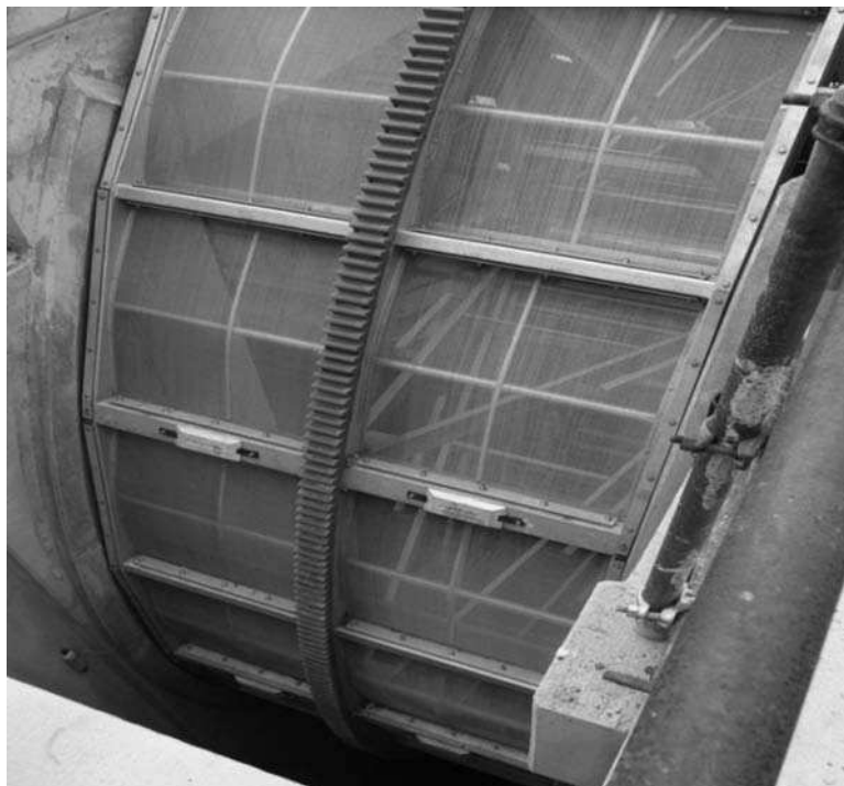
FIGURE 8.5 Drum screen of the Sydney Desalination Plant.
