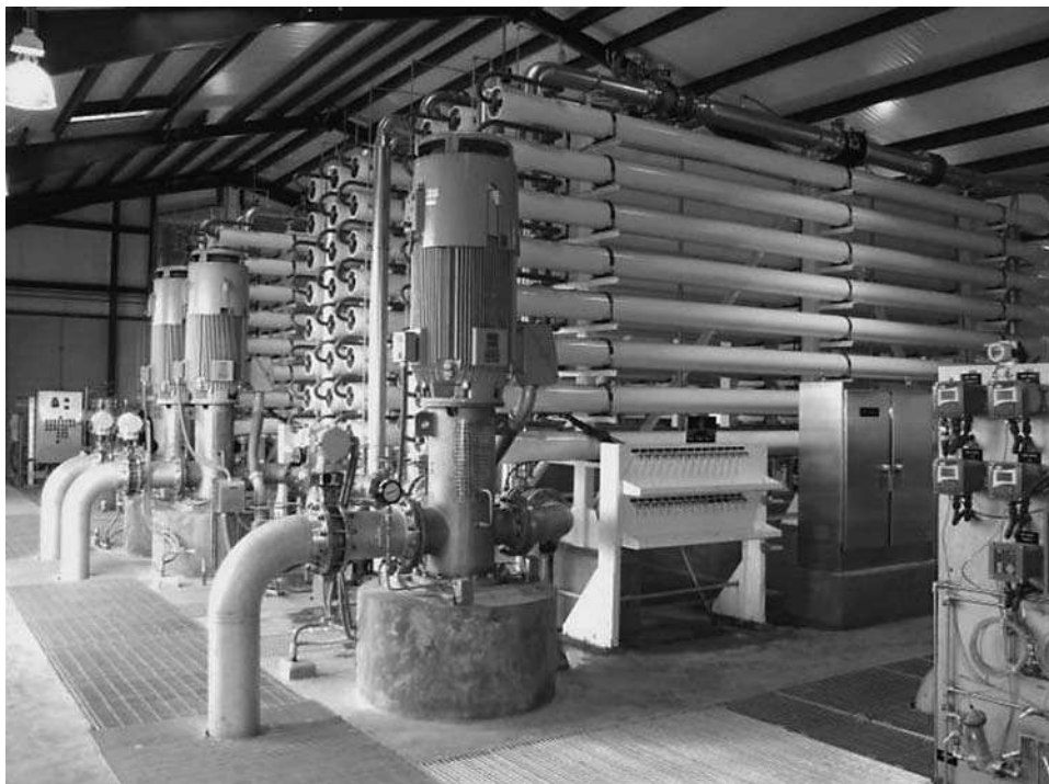
FIGURE 14.6 Vertical turbine high-pressure BWRO pumps.
