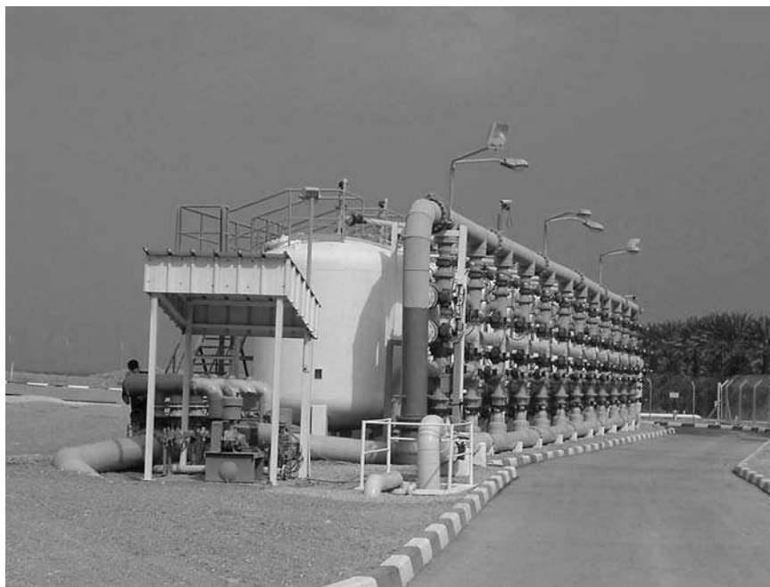
FIGURE 11.4 Vertical pretreatment pressure filters.
