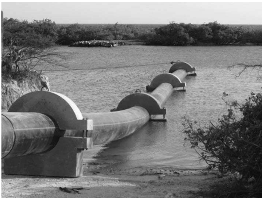
FIGURE 16.4 Outfall discharge pipeline supported on concrete blocks.
