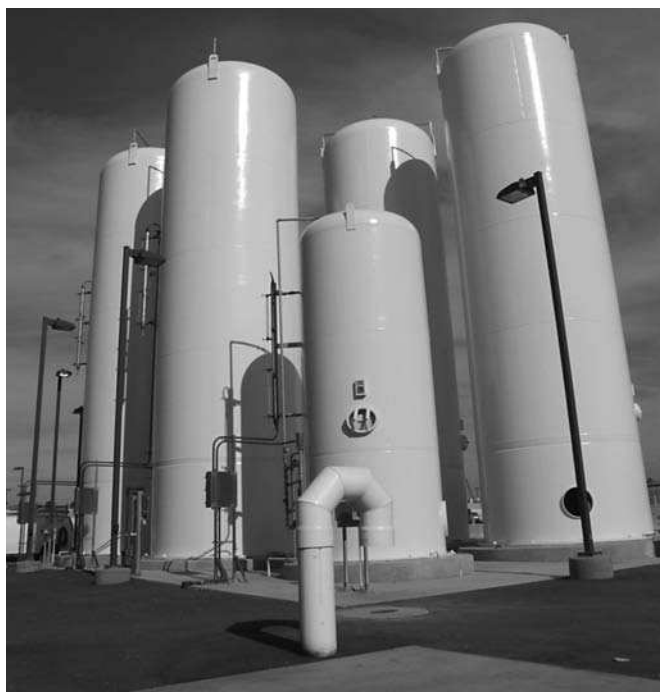
FIGURE 15.4 Carbon dioxide storage tanks.
