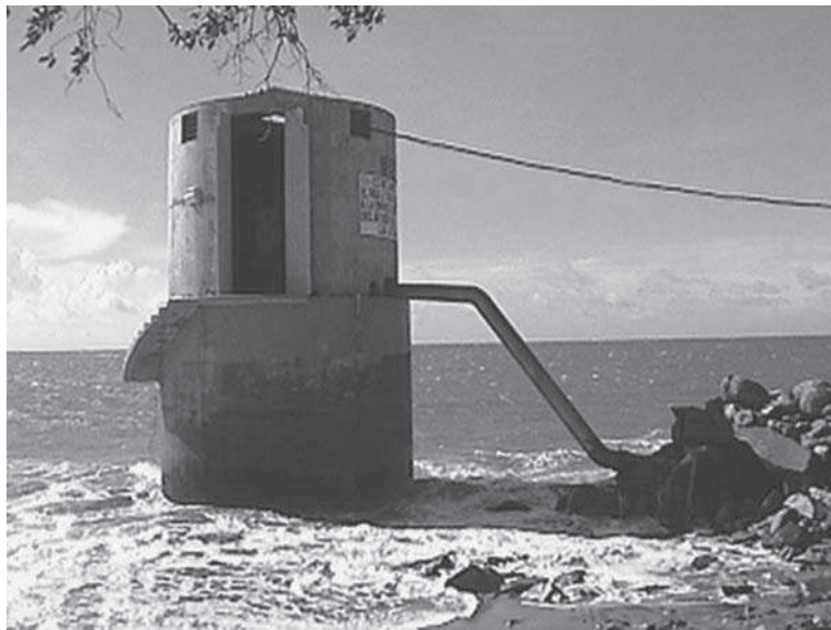
FIGURE 4.2 Seawater intake well exposed to beach erosion.
