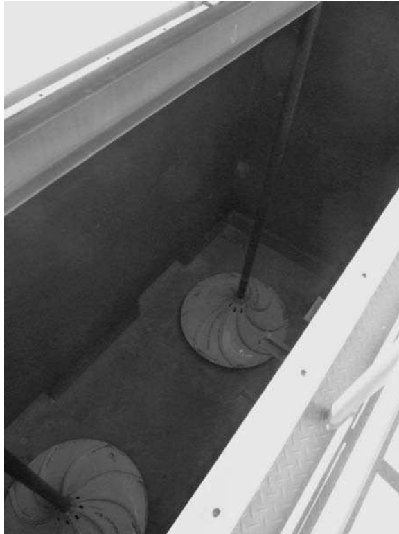
FIGURE 9.2 Flash mixers in coagulation tank.
