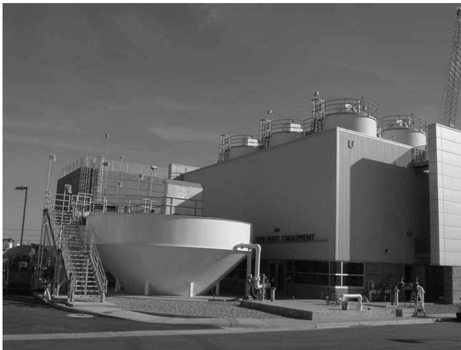
FIGURE 15.3 Lime storage silos and saturator.
