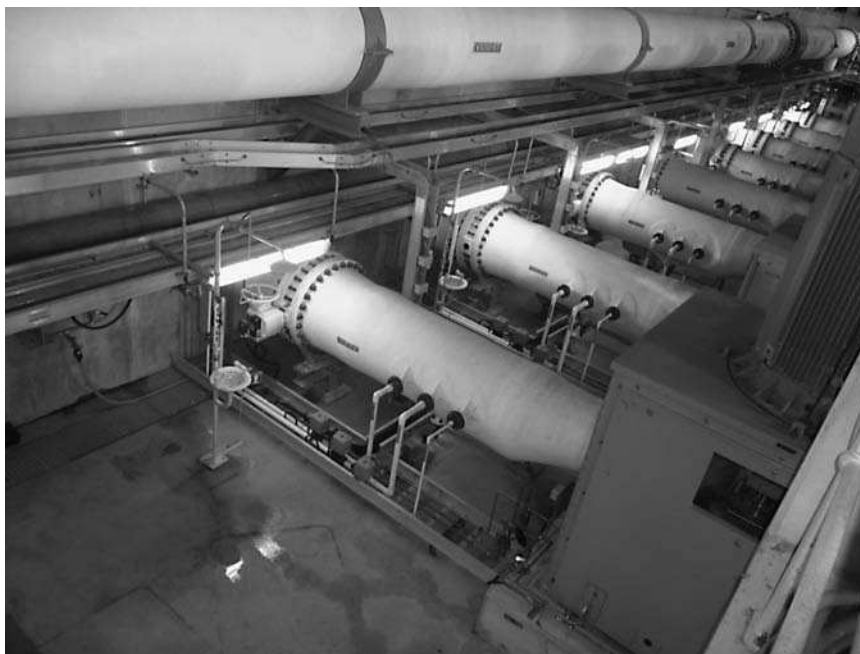
FIGURE 9.6 Point of chemical addition to pretreated water.
