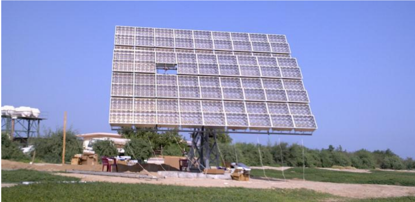
First 10,000 watts Ultra High CPV (UHCPV) at Al Khafji Site
