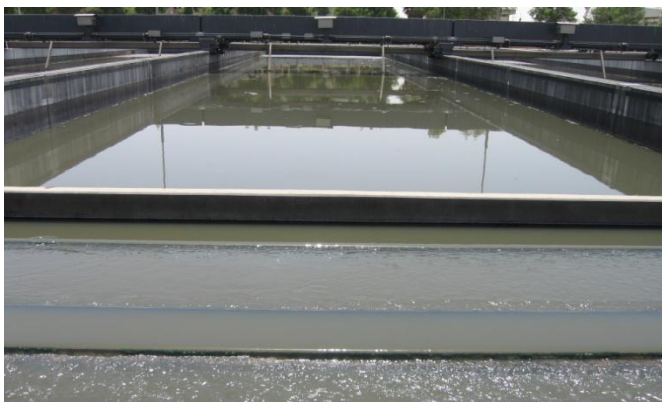
Primary sedimentation tank.
