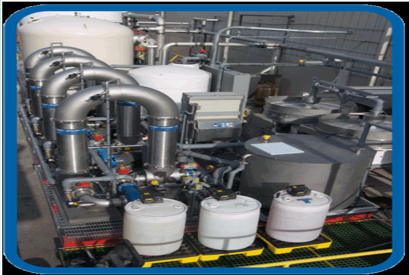
Water reuse reclamation laundry.
