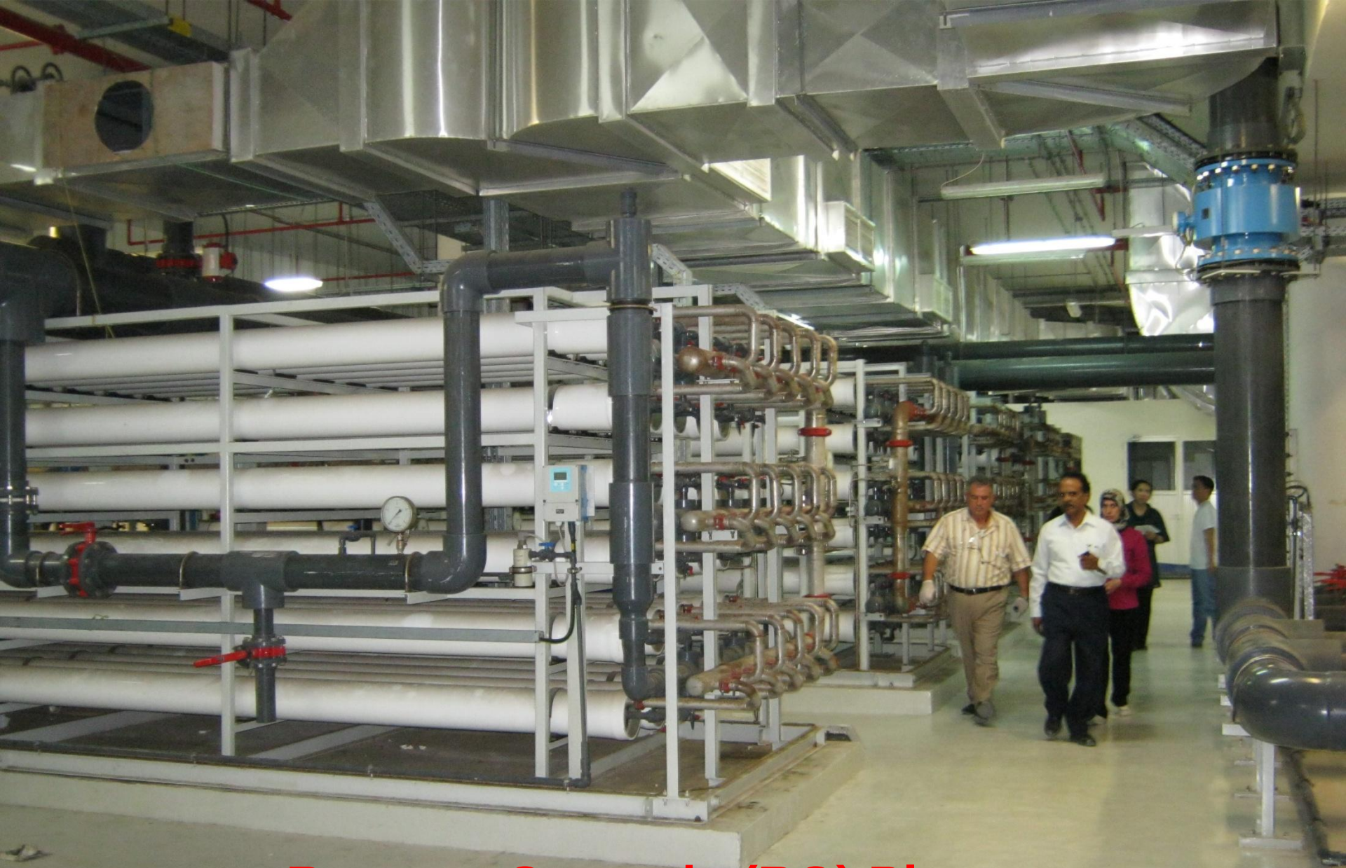
Reverse Osmosis (RO) Plant
