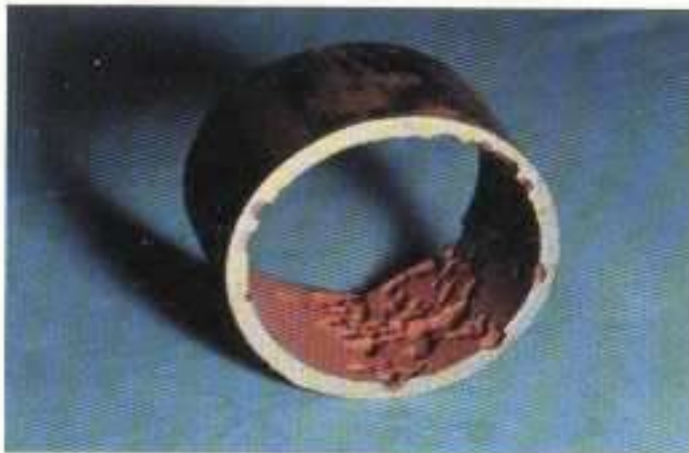
Economizer tube severely damaged by oxygen.
