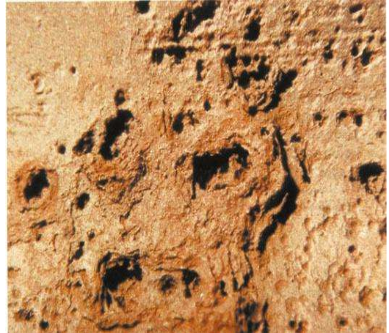
Deposits on turbine before cleaning
