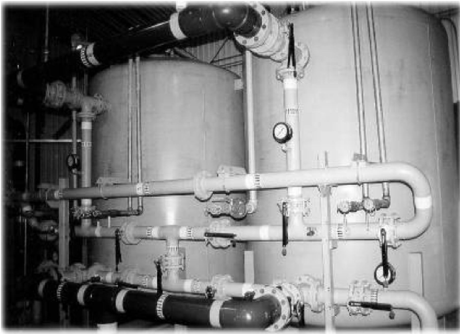
Figure 6.10 GAC adsorption tanks
