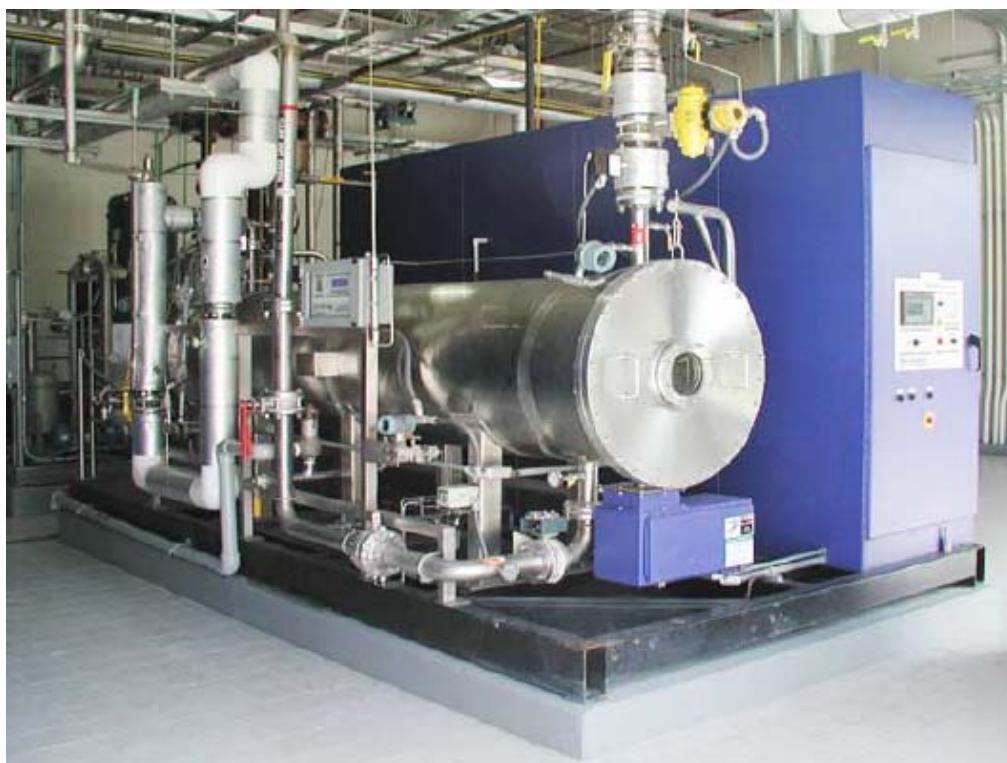
Figure 2.4 – Ozone Generator and Power Supply 2
