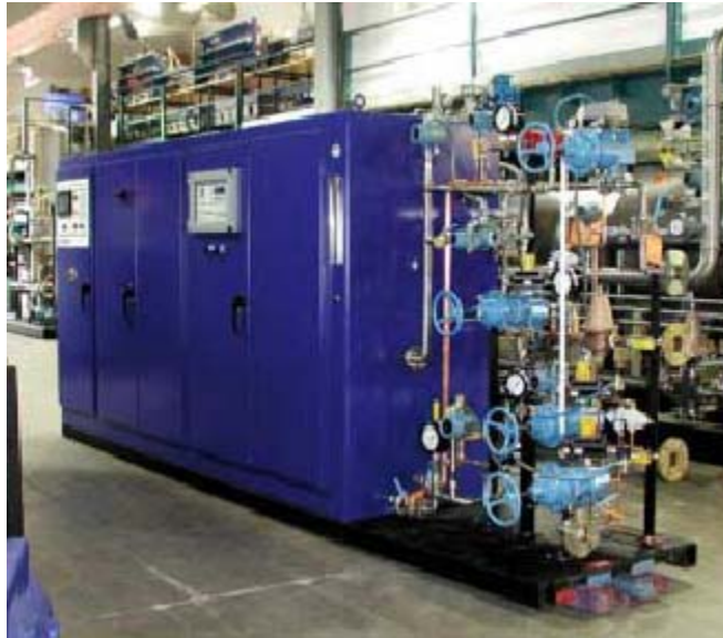
Figure 2.3 – Ozone Generator Power Supply Unit 1
