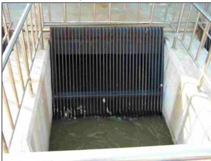
Manually Cleaned Bar Screen
