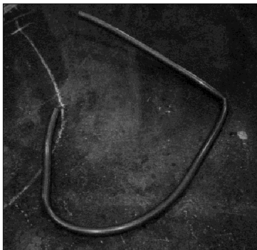
Figure 4.2 Copper tubing incorrectly bent (kinked).
