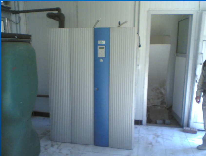
SBR Pilot Plant
