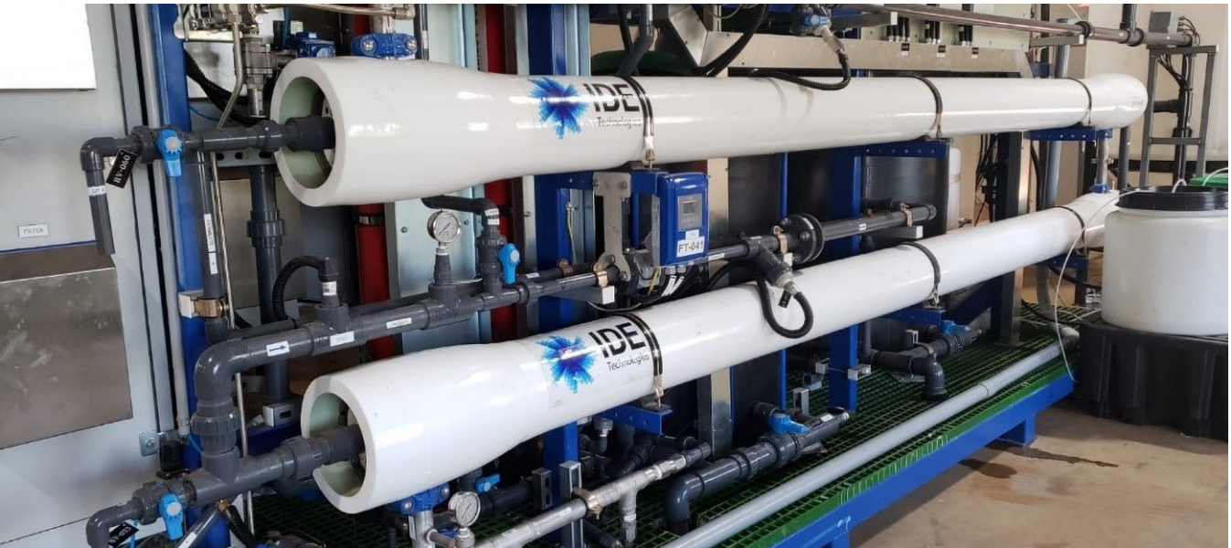
Abilene Hargesheimer Water Treatment Plant
